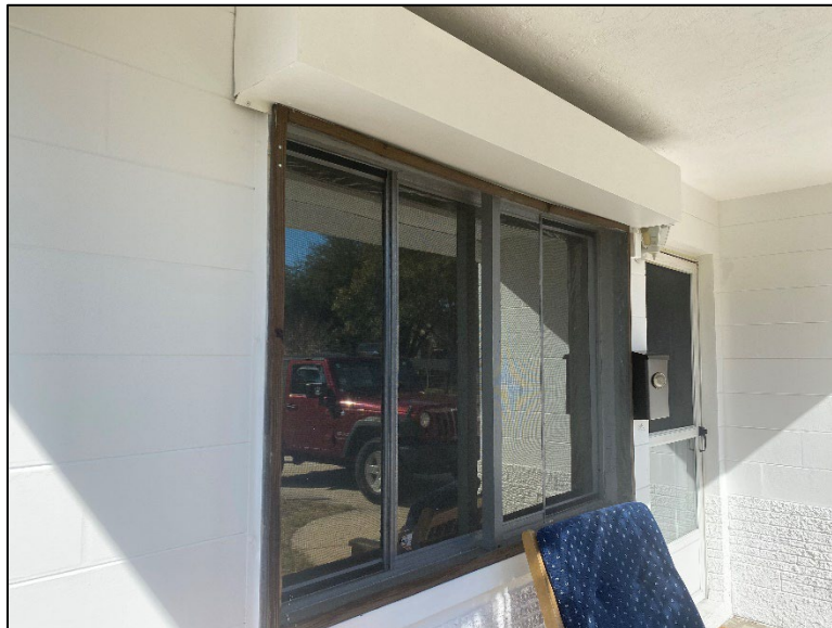
Figure 2: Existing window with roll-down hurricane shutter unit
