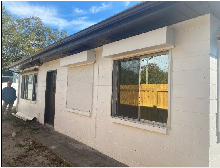
Figure 3: Rear elevation. Window at far left is proposed location of sliding glass door.
